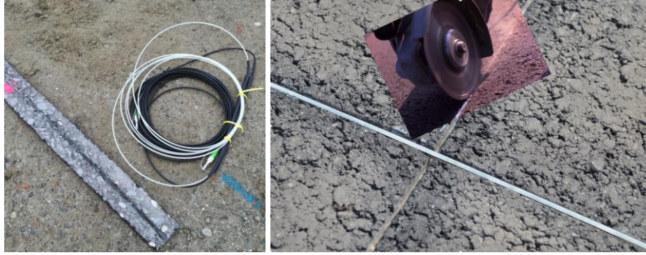
FIGURE 2 Installation of FBGs in prefabricated asphalt in base layer (a) and installation of FBGs in the previously constructed asphalt layer (b)
